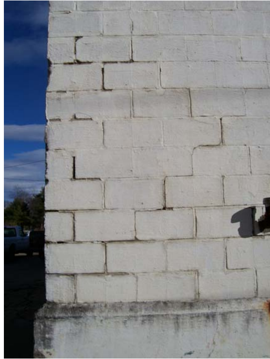
Photo 3. Cracks in masonry
